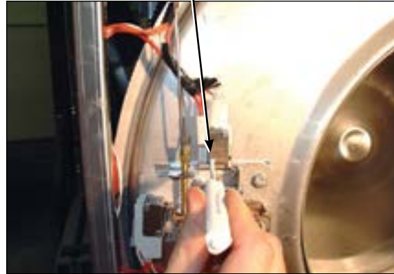
Flat blade screw on door switch latching
