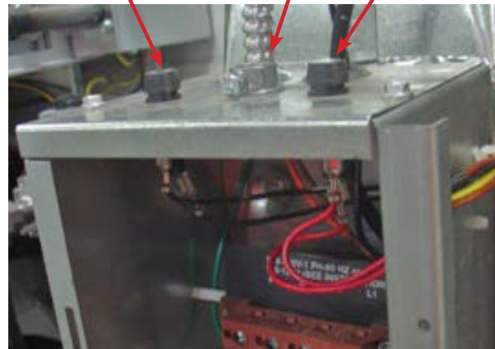
Control Protection Fuse 2.5 Amp 14 1 Ignition Upper Pocket Protection Fuse 1.5 Amp 14
