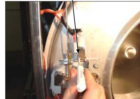
Flat blade screw on door switch latching
